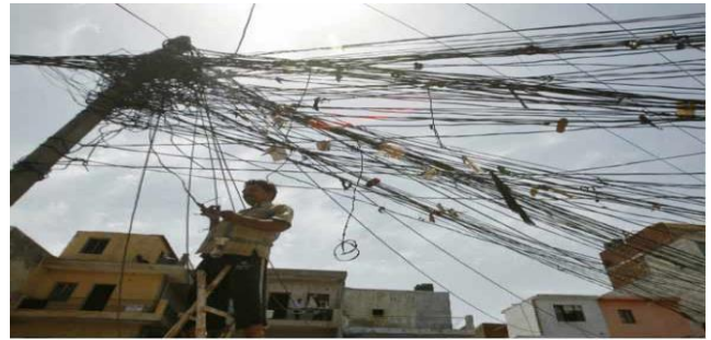
A man stands on a step ladder to fix tangled overhead electric power cables at a residential area in Noida, India, June 1, 2011 (Parivartan Sharma/Courtesy Reuters).
