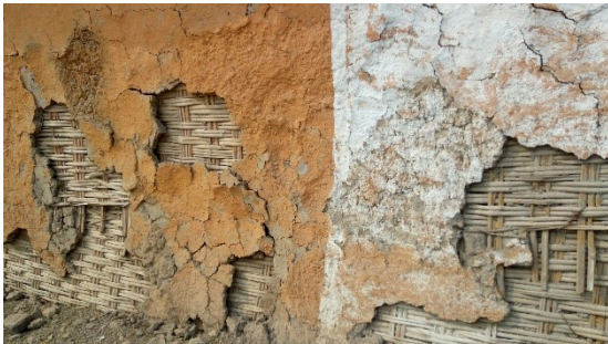
Figure 1. Wall succumb due to rain fall
