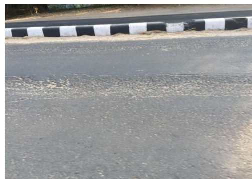
Figure 2. Rutting on Road of SH-158
