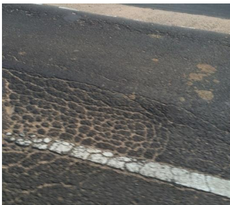
Figure 5. Alligator Cracks on Road of SH-158
