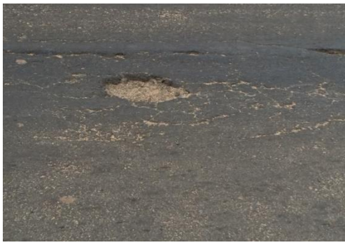
Figure 3. Pothole on Road of SH-158
