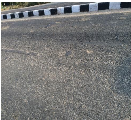
Figure 6. Hungry Surface on Road of SH-158
