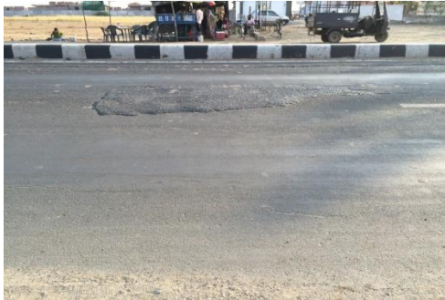
Figure 4. Patching on Road of SH-158
