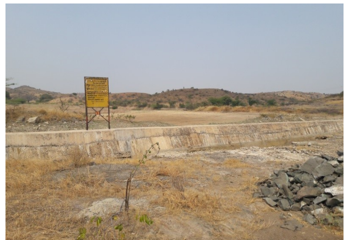
Figure 5. Check dam in khor village
