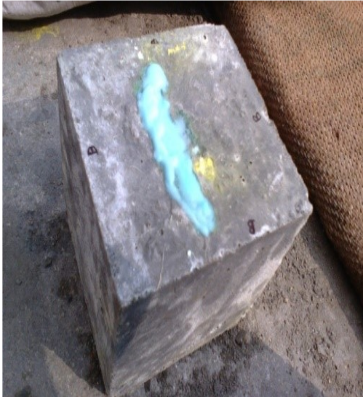
Figure 9. Crack filled with solution with bacteria
