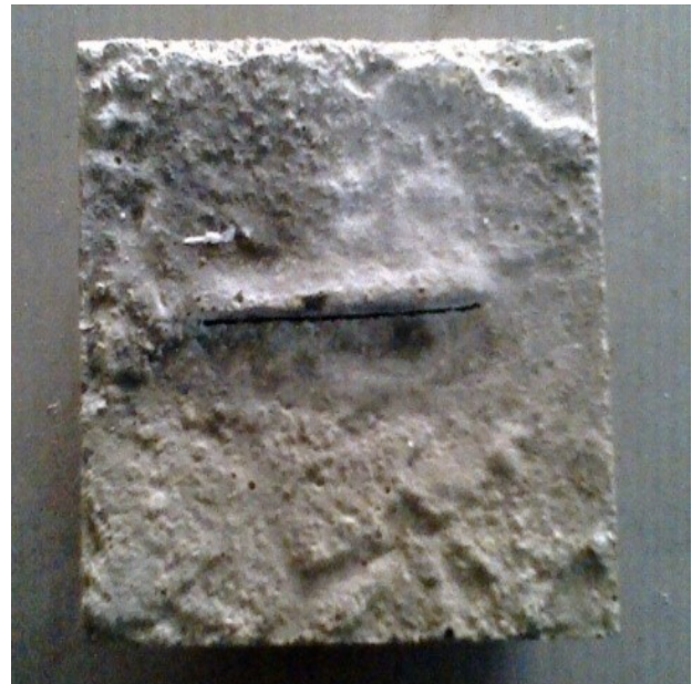
Figure 7. Crack formed on the surface
