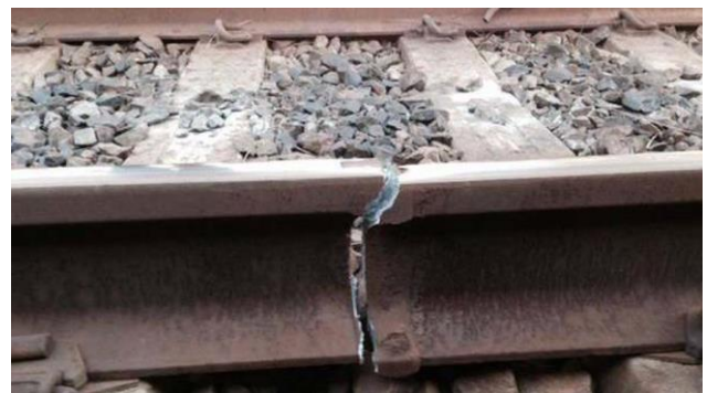
Figure 1. Cracks in Railway tracks
