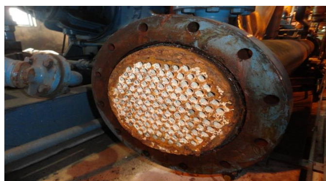
Figure 1. Vacuum pump cooler found outside corrosion on outer surface and inside tubes
