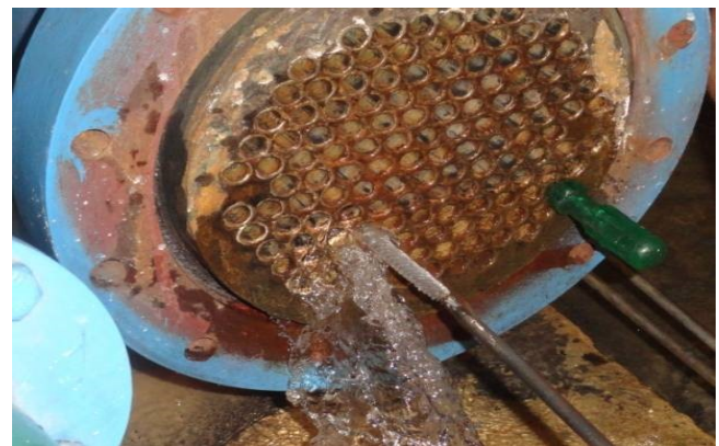
Figure 3. vacuum pump cooler cleaning by high pressure jet and mechanical brush cleaning
