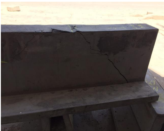
Figure 4.3: first Crack simple A 1
