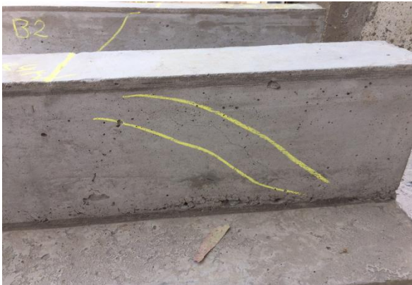
Figure 4.2: first Crack simple A 2
