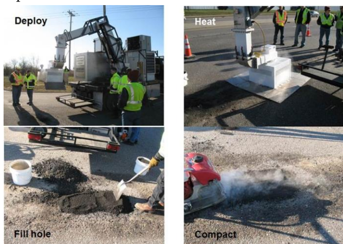
Figure 1. Patch work of road
