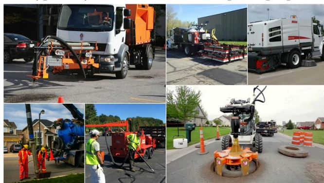
Figure 2. patch work of road
