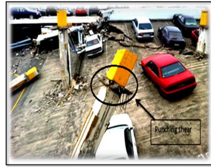
Figure 4. Punching shear failure
