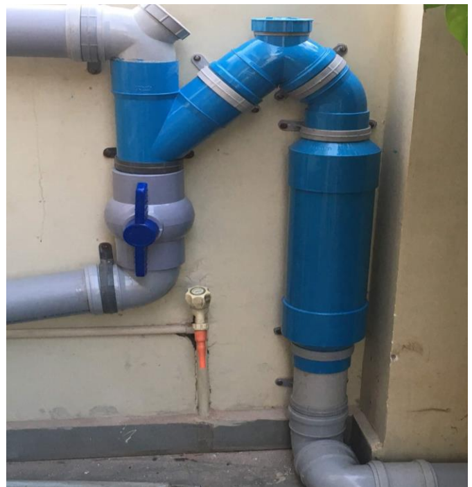
Fig 8. Installed rainwater harvesting filter
