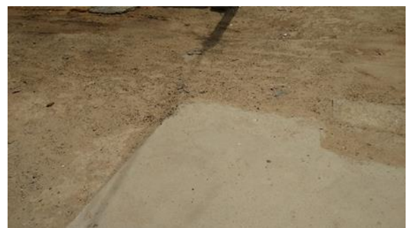
Figure 4 : Poor road condition in village.
