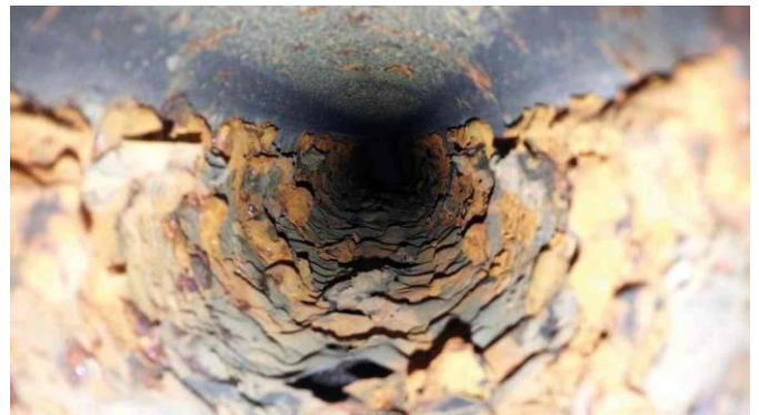
Figure 1: Severe corrosion inside steel pipe of a wet type fire sprinkler system (image by IFP: The problem of corrosion in metal fire sprinkler system 2017
