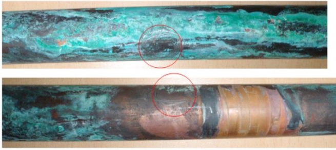
Figure 2: Corrosion failure copper tubes, red circles display water leakage locations [44]
