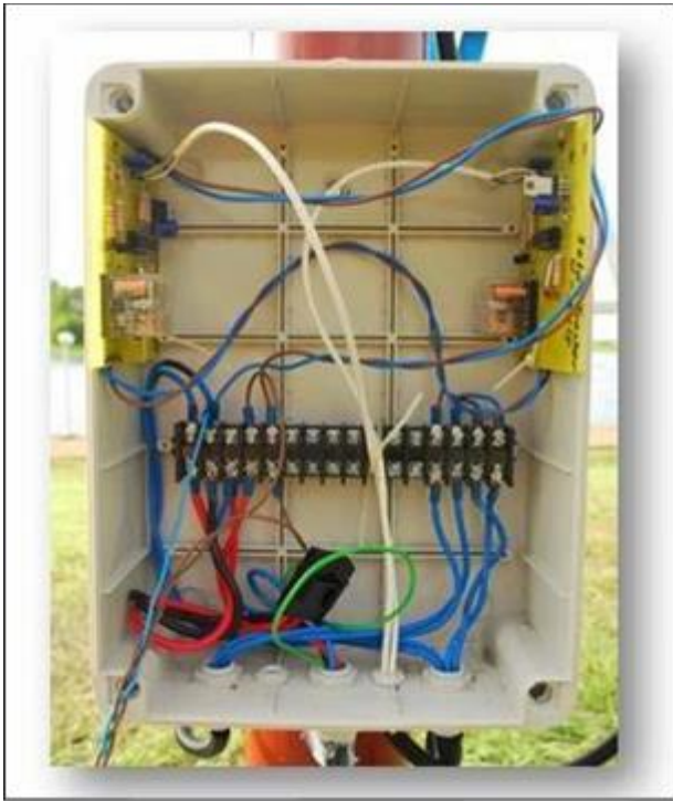
Figure 16. Inside the controller box.
