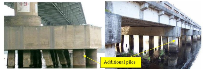
Figure 18. Addition of piles applies to the case that the abutment foundation of the bridge in the downstream area of Vam Co river is not able to bear the load and additional piles are needed.
