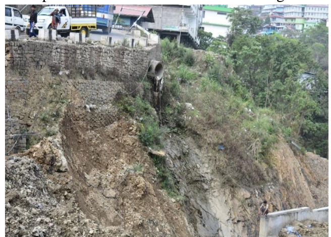
Plate 3: Landsliding along the bank of the river Sano ru.
