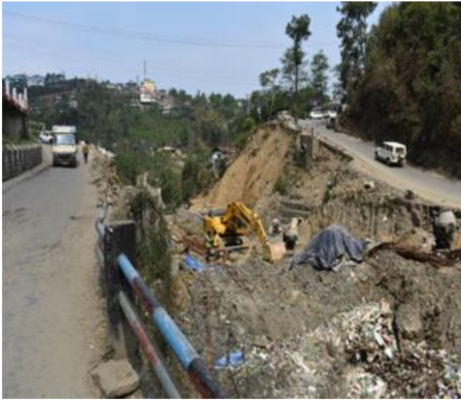
Plate 4: Landslide and subsidence along Sano ru, where a road connects the Secretariate with the rest of the district
