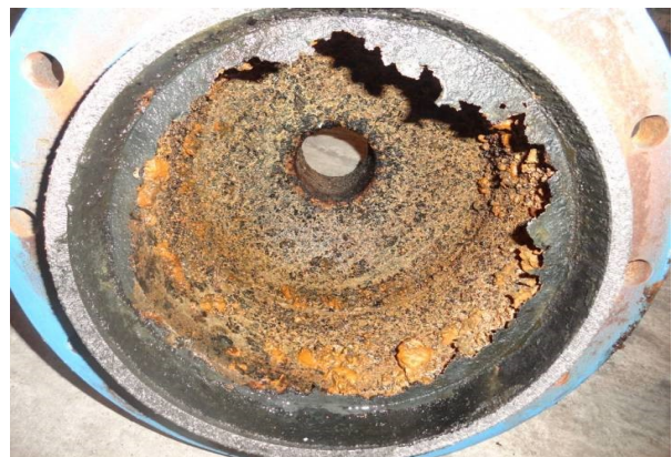
Figure 2. vacuum pump cooler tubes fouling with corrosion on cooler dome
