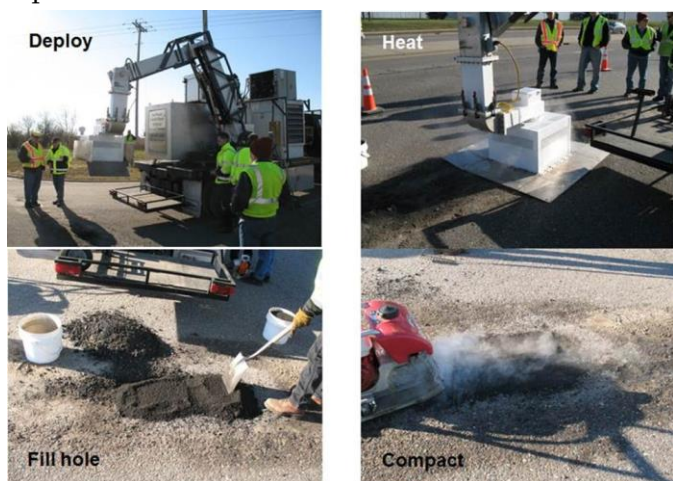
Figure 1. Patch work of road
