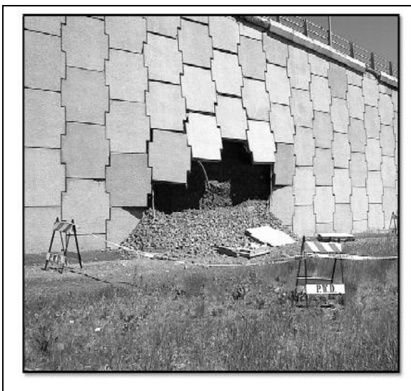
Figure 3. Failure Of Retaining Wall
