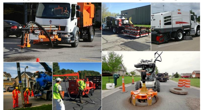
Figure 2. patch work of road
