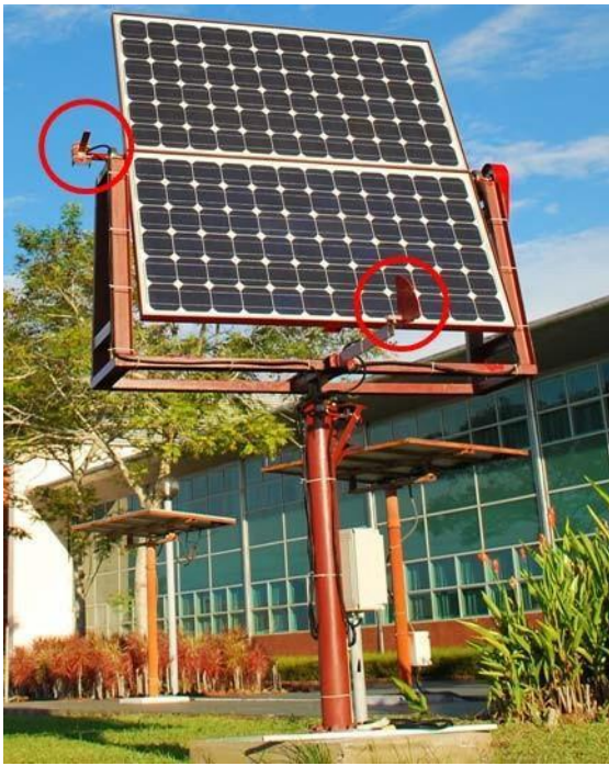
Figure14.Placement of the sensoron thestructure.
