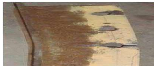
Fig. 4.2 Partial net section ruptures, with large eccentricity
