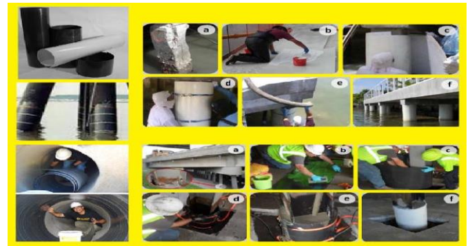
Figure 16. Using prefabricated FRP sheet (a). Prepare the FRP sheet; (b) Construction of FRP sheets; (c) Fixing and finishing the FRP sheet; (d) High strength grout pump, (e) After finishing
